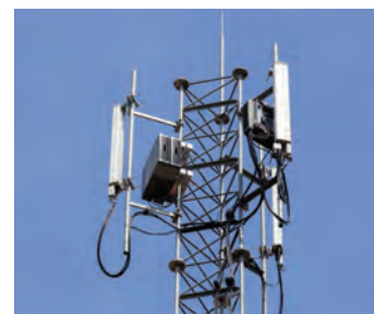
Mobile Tower Switching Areas
